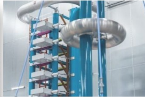
High Voltage Substation Equipment
